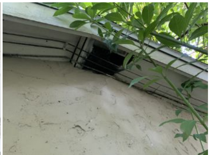
Hole in ev
