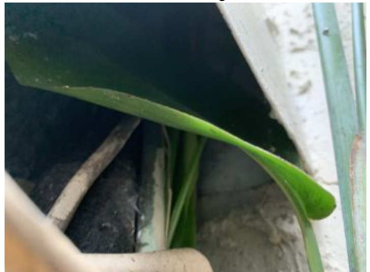
A/C Chase is not sealed. This acts as a highway for rodents and insects
