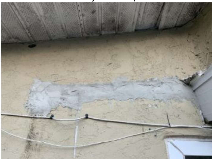
Stucco repair requires sealing and paint
