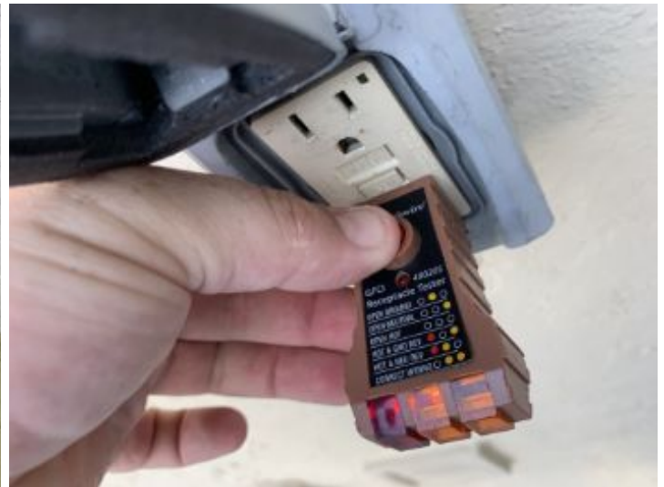
GFCI Trip fail, wired incorrect
