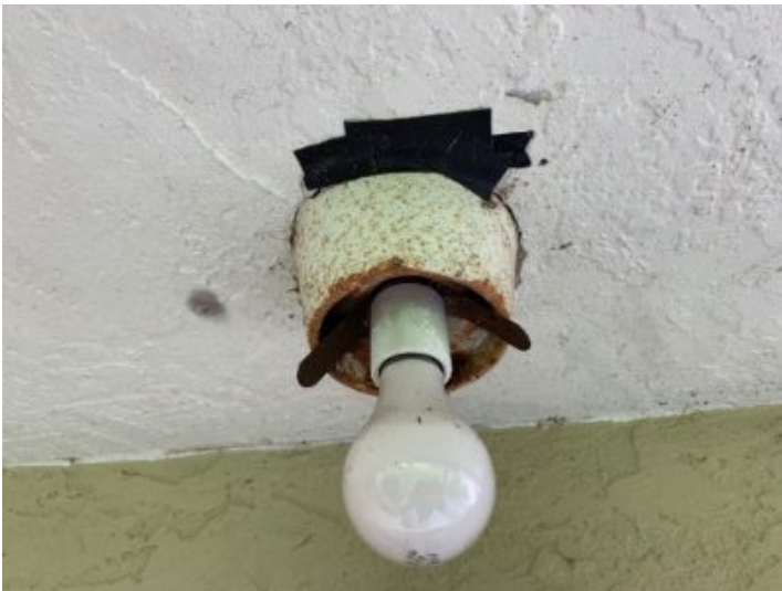
Exterior lights rated for interior
