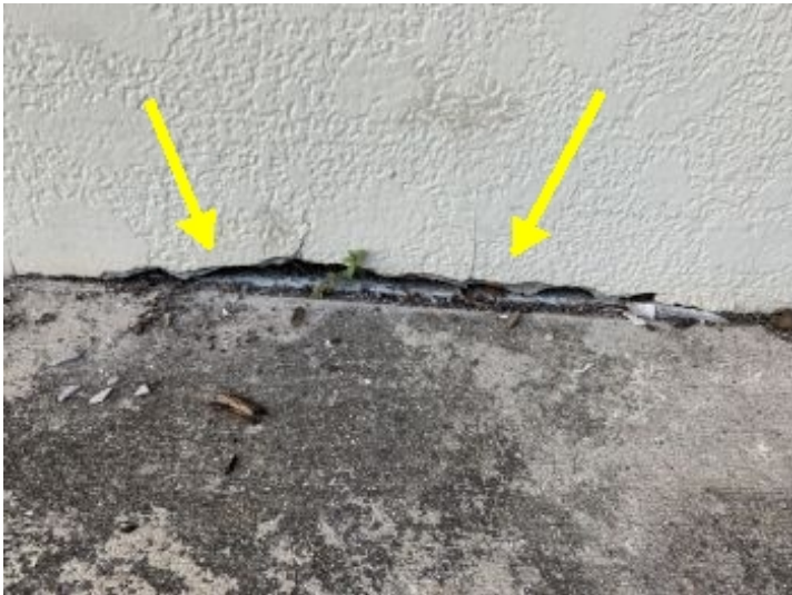
Hardi board used as siding for front storage area. Bottom is broken and starting to deteriorate
