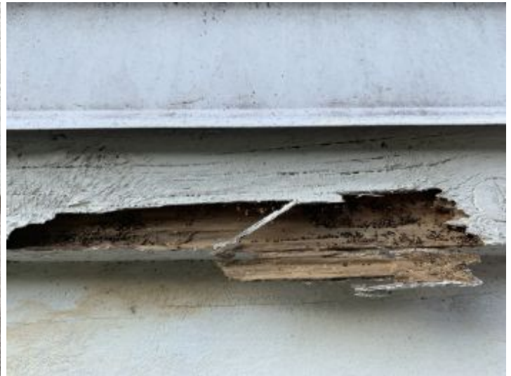
Some wood deterioration noted at front eave trim. Have repaired and inspected for wood-destroying insect damage.
